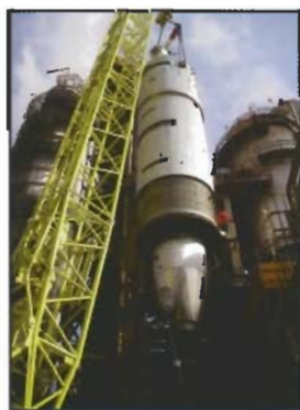
Large lifts and installs such as this are rehearsed using 3D autocad to make sure things will be done right the first time and all will fit correctly.
