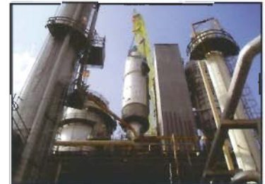
Difficult projects are a specialty at AltairStrickland. Experienced personnel and planning are the key to successful project such as this.
