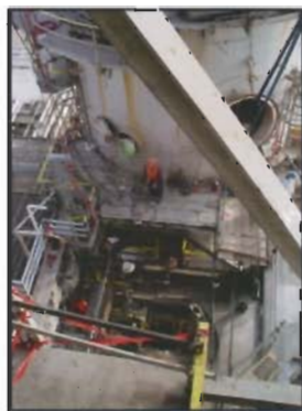
As much structure modification as possible is done ahead of time to reduce the unit downtime. AltairStrickland utilizes Certified Safety Specialists, a third party safety provider for their safety professionals and attendants.
