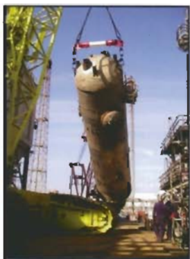
By calculating and planning ahead of time the risk is taken out of big lifts such as this, downtime is minimized and safety is put at the forefront.
