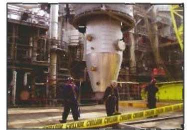
AltairStrickland riggers make sure the rigging lines up correctly for the installation.
