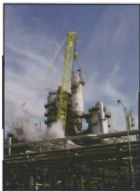
Crane selection for your project can be crucial. AltairStrickland's engineering and project team helps the customer by bringing the experience of over 28 years of heavy lifting and knowledge of recent innovations within the industry to help save the customer time and money during the project.
